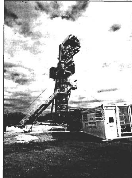
Fig. 1. A fully integrated slimhole drilling rig uses the same tubing handling system to drill with coiled or jointed tubing.
